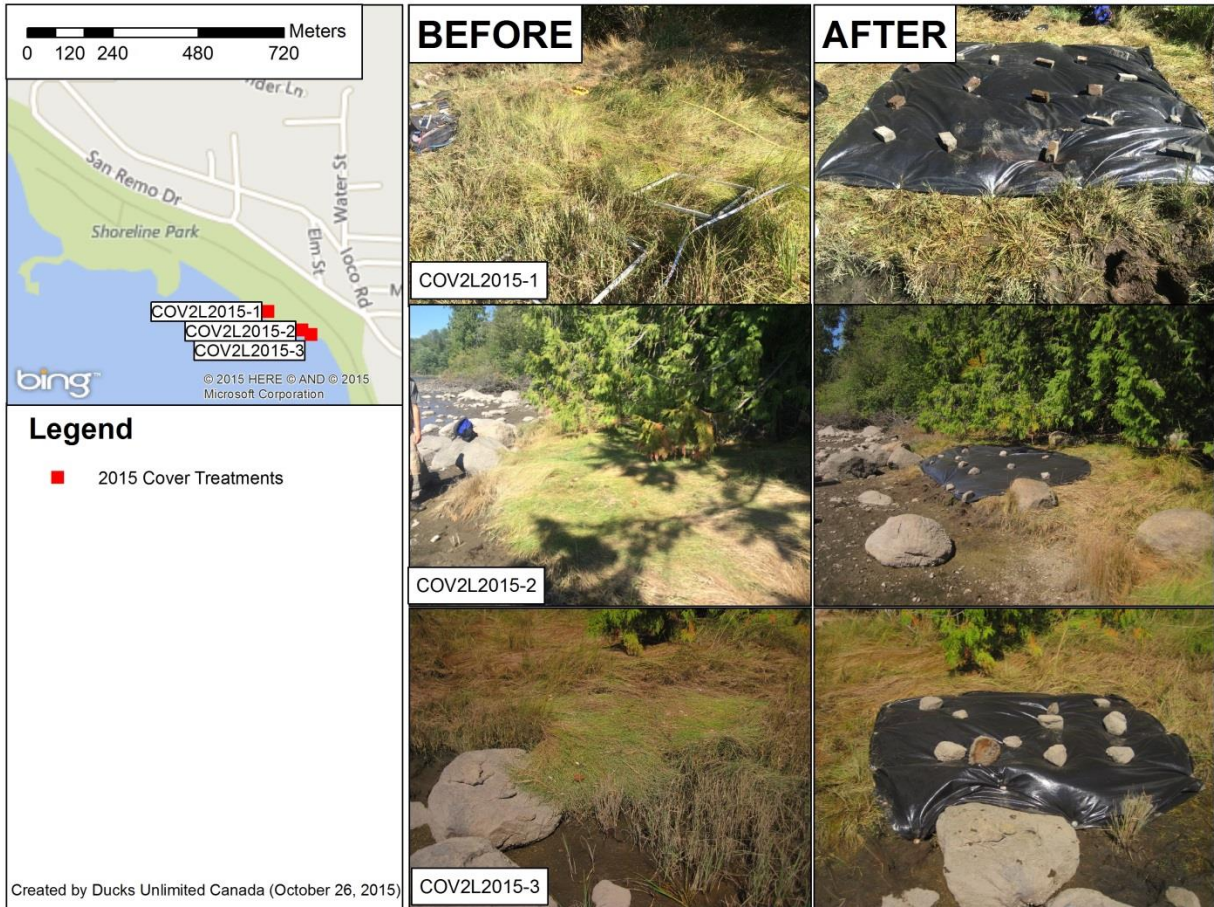
Figure 16. Locations and Before/After photos of three cover plots installed in Port Moody in August 2015
